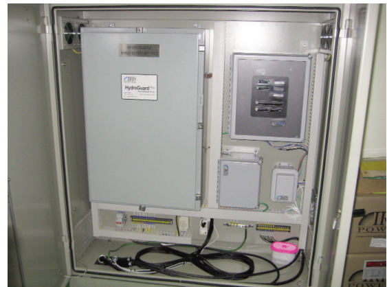
Installation of the FluxTrac//S (right side) as well as the HydroGuard PD monitoring system in a hydrogenerator plant in South Asia.
