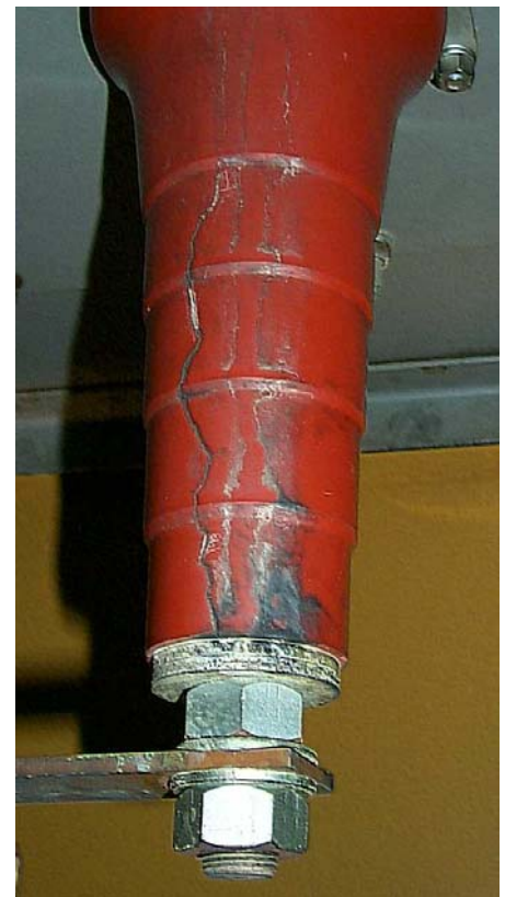
Figure 2. Heavily tracked generator bushing (photo taken after cleaning)
